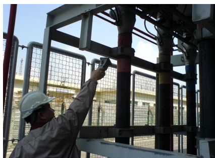
Figure 2 : Overhead cable PD test
