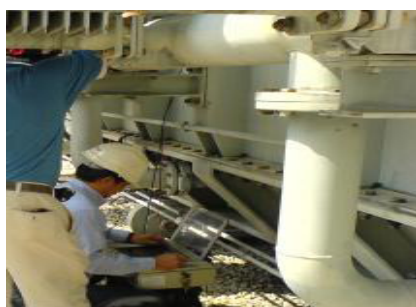
Figure 5 : Oil type transformer PD test
