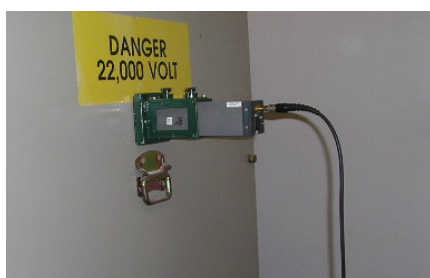
Figure 3 : Switchgear panel PD test
